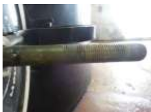
Threaded bolt showing wear
