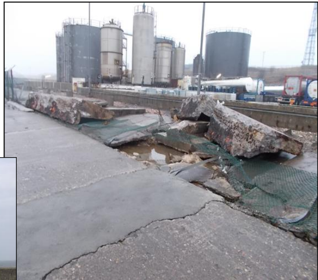
Above - Picture of the damaged wave guard (photographed from the seaward side)
