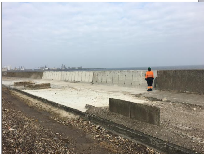
Left – Picture of the repaired wave guard (photographed with the site behind the camera)
