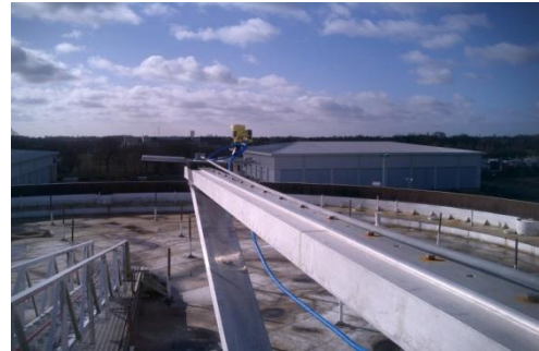
Automated system for preventing tank over-fill Picture Source: UK Petroleum Industry Association
